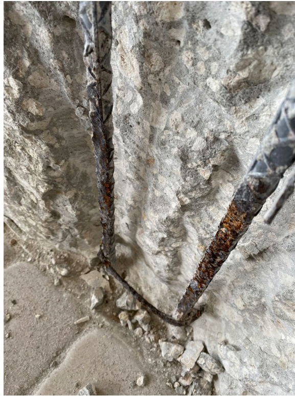
Picture 5: Typical corroded and necked down reinforcing steel in garage
