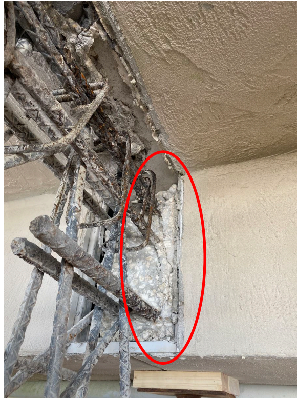
Picture 3: Cracked concrete at beam going above garage soffit
